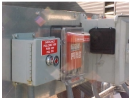
8) Skyport fuel shut-off, fire alarm pull station and outside telephone box
