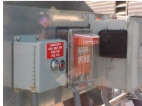
6) Fuel shut-off, fire alarm and phone
